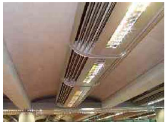
FIGURE 4: Chilled beams can be integrated with lighting.
